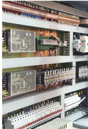
电箱 Electric box
